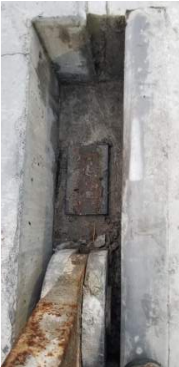
Crane Tie-Down Vault with no drain.
