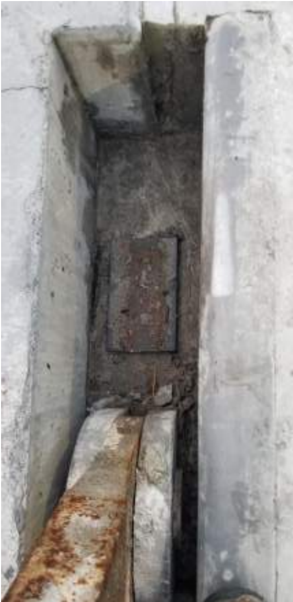
Crane Tie-Down Vault with no drain.
