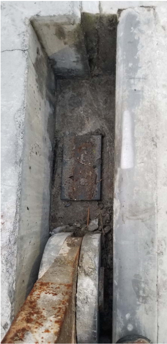
Crane Tie-Down Vault with no drain.
