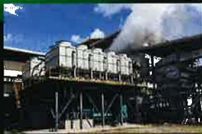
Kaishan geothermal power plant in Indonesia
