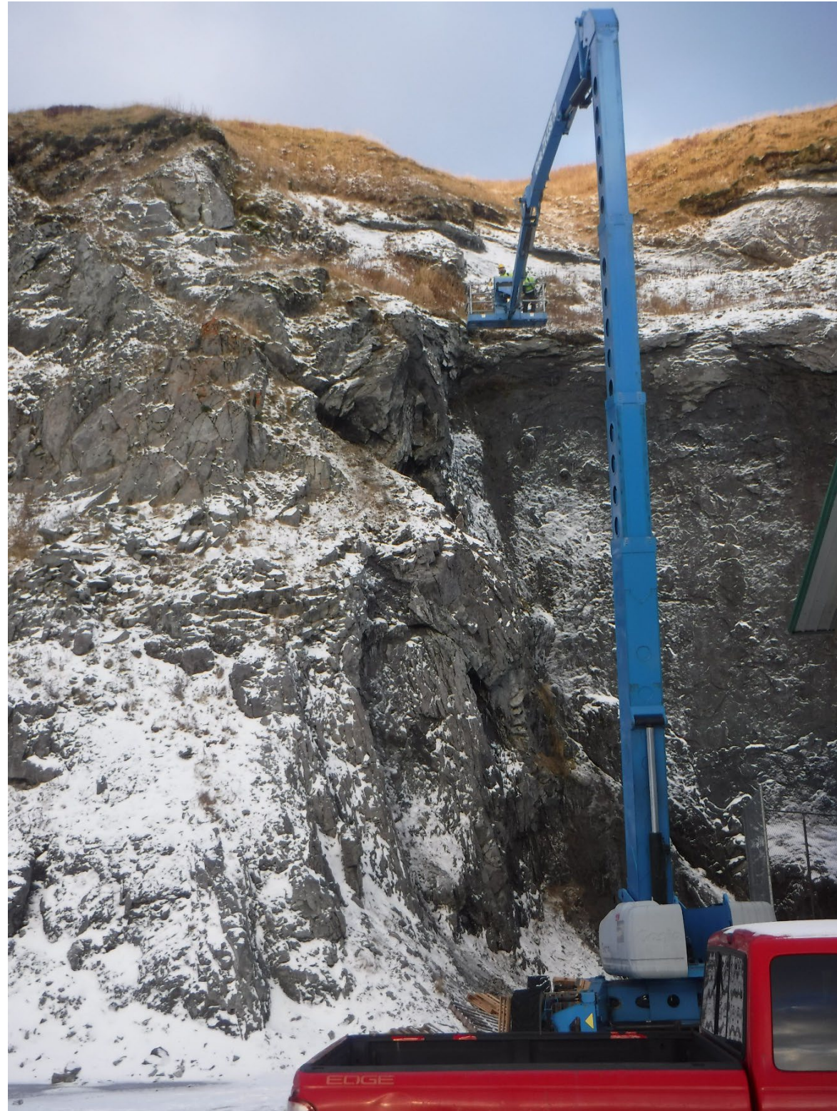
Description: Day 1 Scaling Operations at WU 1a Via Manlift Photo Date: Dec 05, 2023
