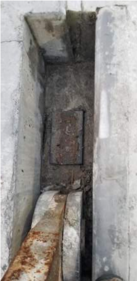
Crane Tie-Down Vault with no drain.
