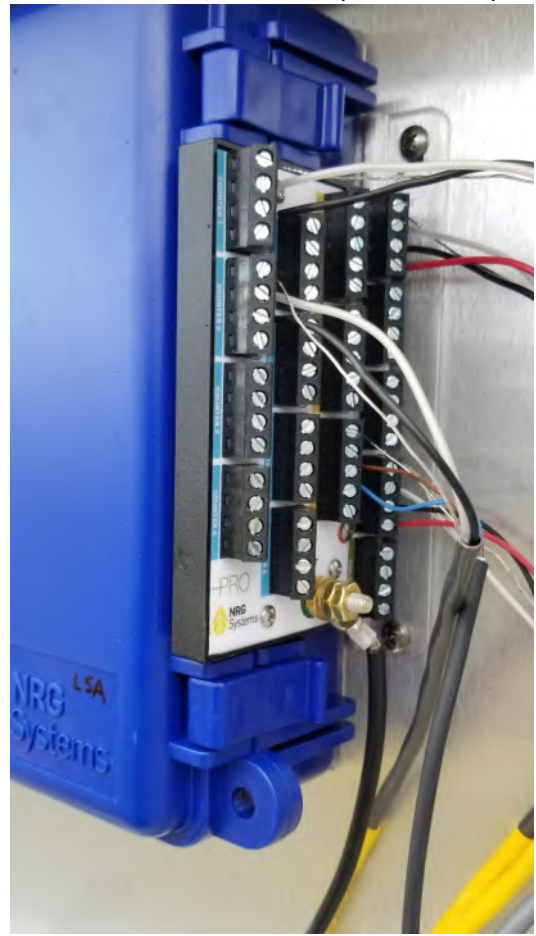
Bunker Hill 10 m, datalogger wiring panel
