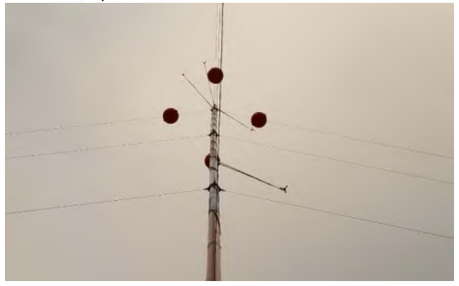
ICR 34 m, uptower, southwest face
