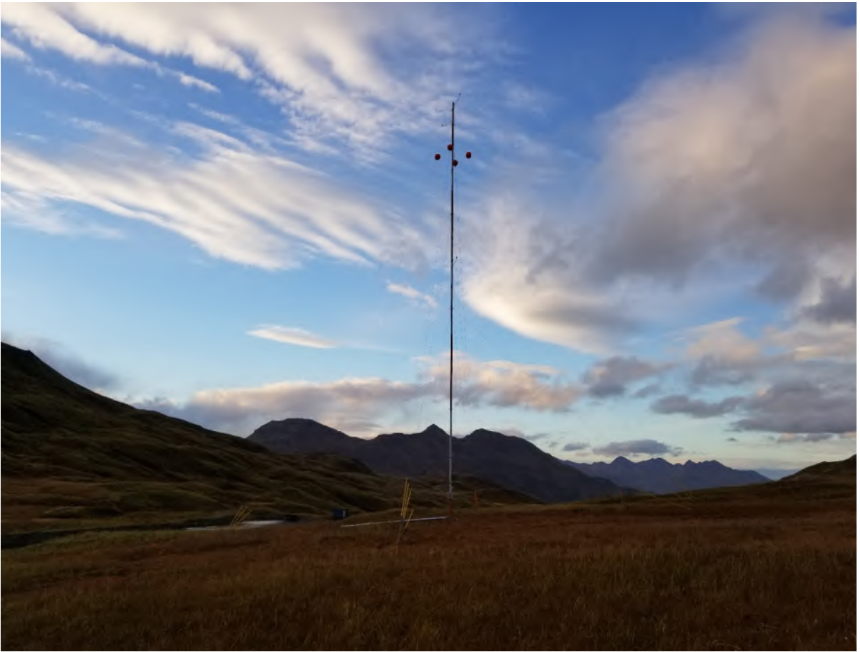
ICR 34 m met tower, view to northwest
