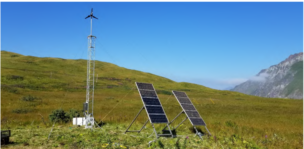
Hog Island 60 m, power system for lights
