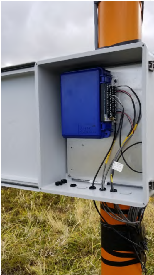
Bunker Hill 10 m, weather box
