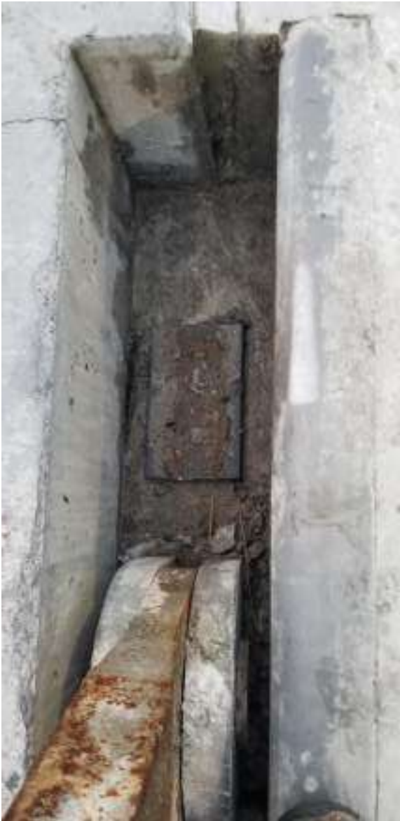
Crane Tie-Down Vault with no drain.
