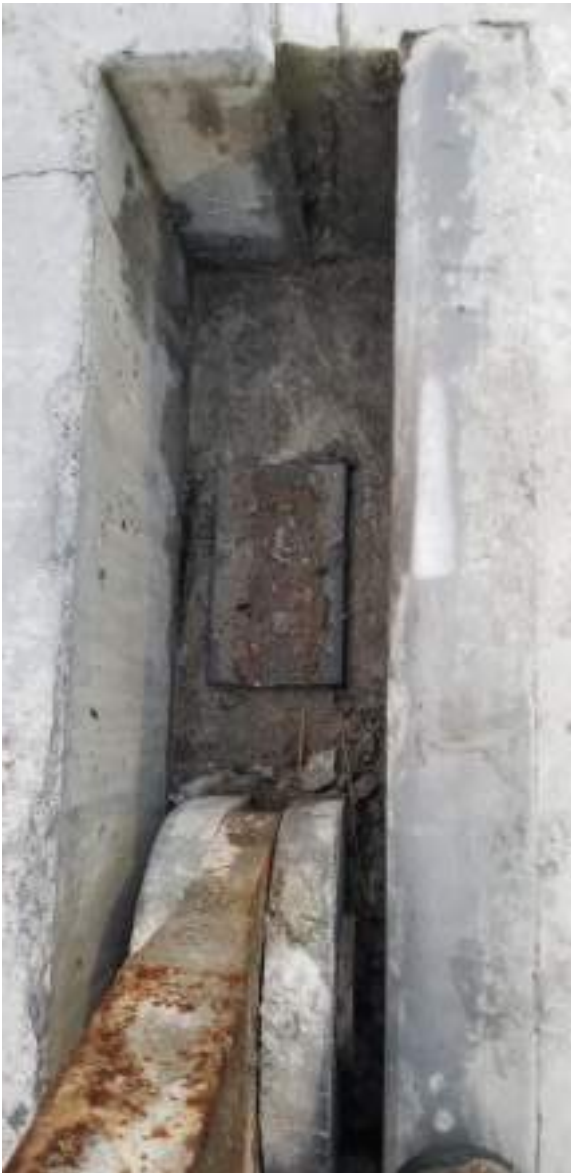
Crane Tie-Down Vault with no drain.
