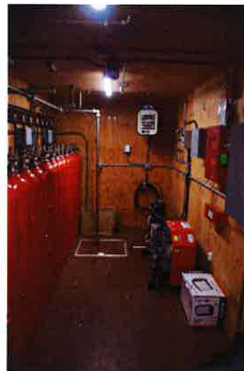
Fire suppression system pressurized canisters in conex.
