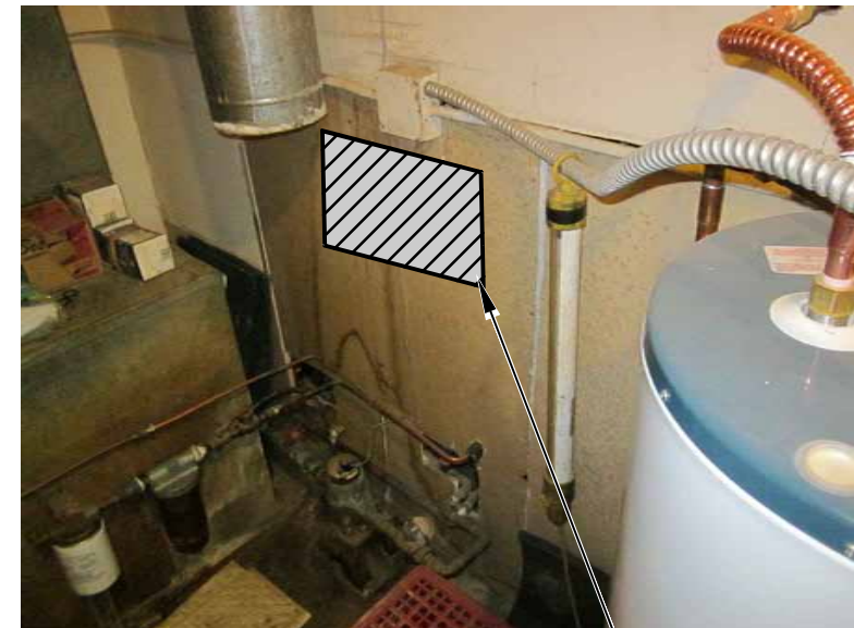
1 5.08 PHOTO SCALE: NOT TO SCALE INSTALL RPBA THIS AREA, ROUTE DRAIN ALONG WALL TO BUILDING EXTERIOR
