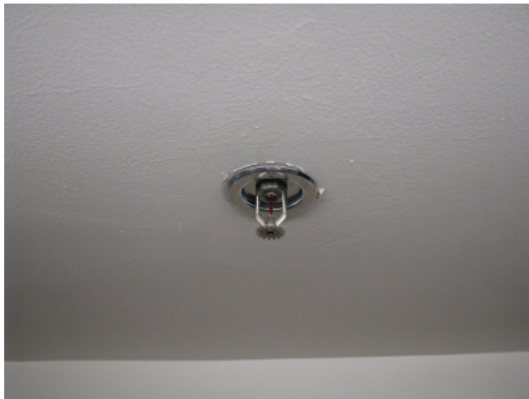
IMAGE 1. SPRINKLER HEAD LOCATED IN MEN'S LOCKER ROOM
