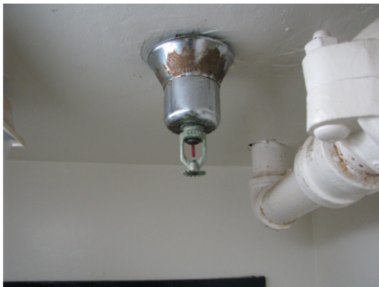
IMAGE 2. SPRINKLER HEAD LOCATED IN HALL 109
