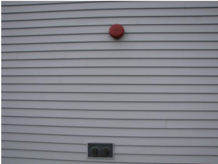
IMAGE 8. EXTERIOR FIRE ALARM AND FDC
