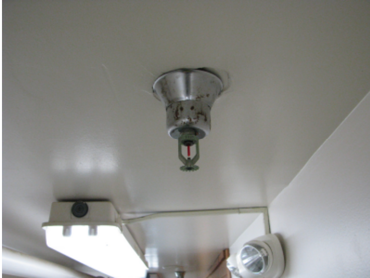
IMAGE 3. SPRINKLER HEAD LOCATED IN HALL 109
