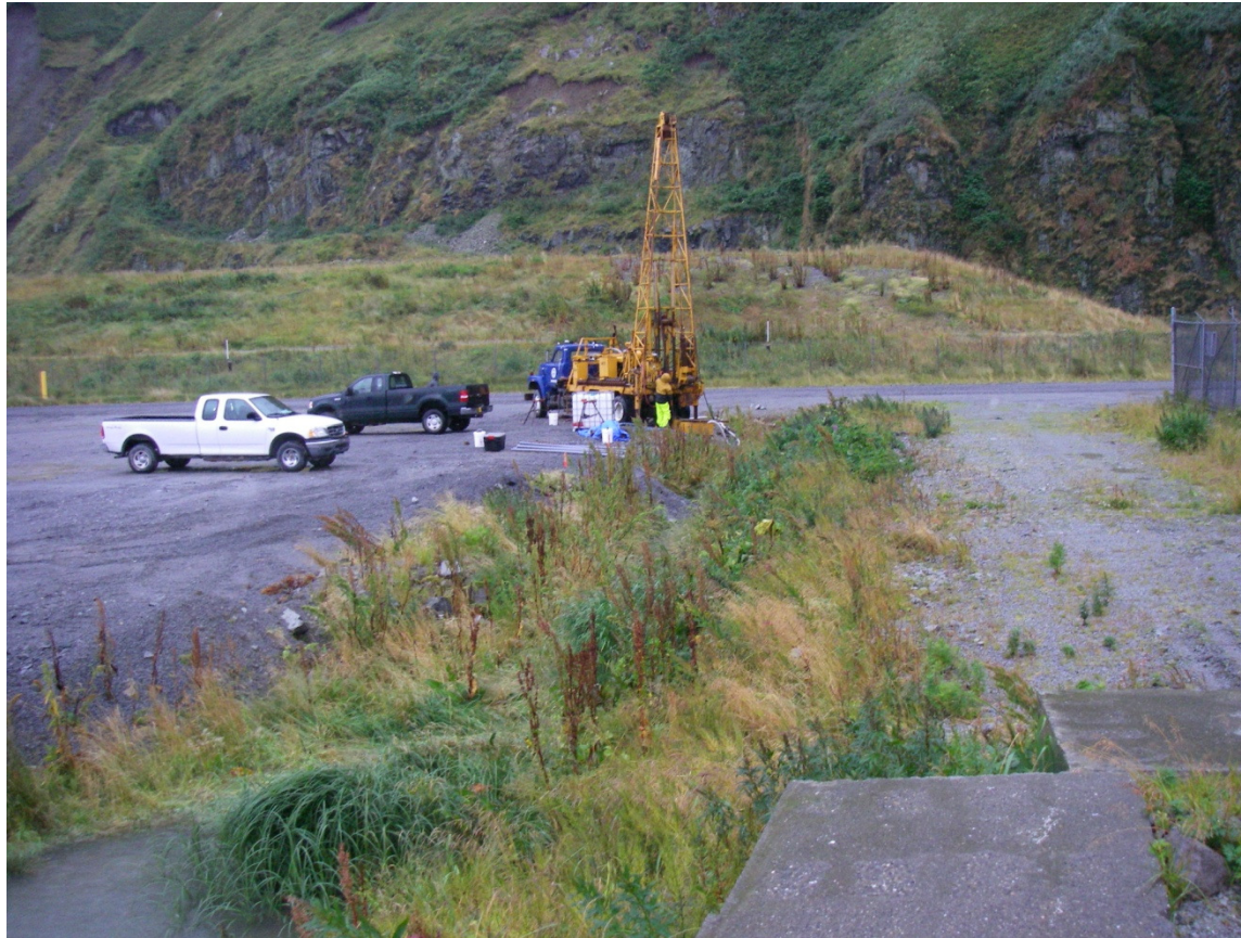
View east up drainage ditch at preferred tank site. Drill rig on borehole G10-BH01.
