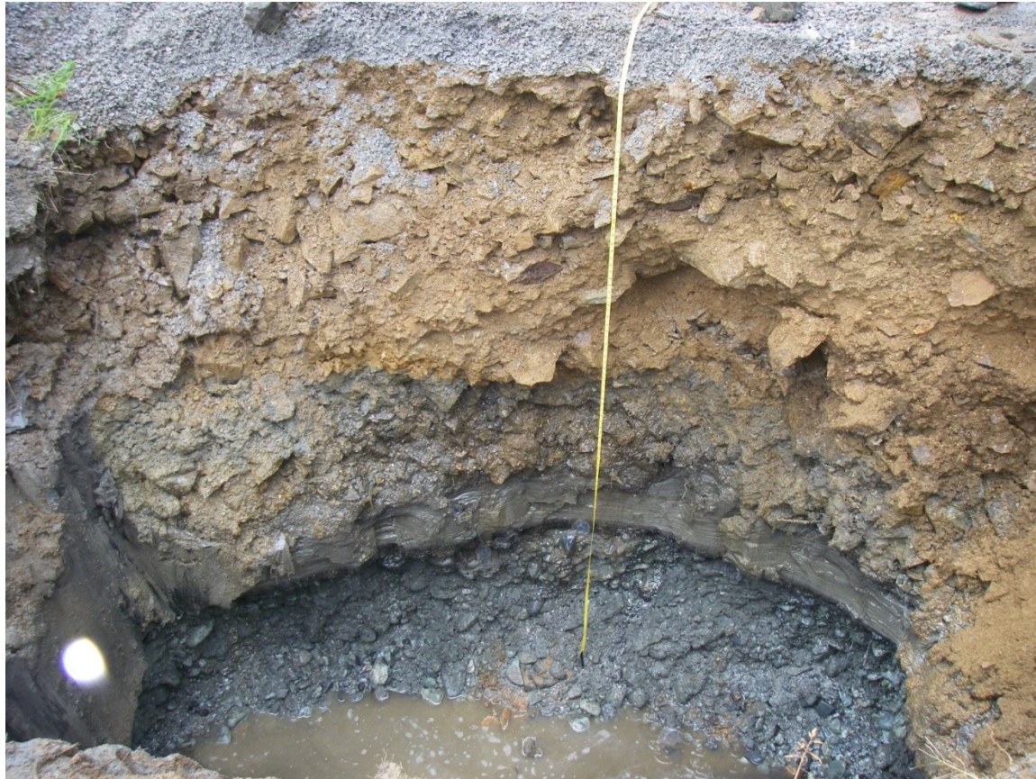
Completion of test pit G10-TP01 at 11.5 feet depth. Note horizontal, gray, high plasticity silt and clay layer in lower third of photo, underlain by “beach gravel” at bottom of test pit.
