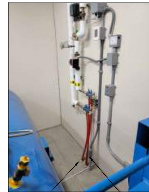
FULLY ENCASE EXISTING LINES IN NEW CONTAINMENT WALL RELOCATE PULLBOX TO ABOVE NEW CONTAINMENT WALL
