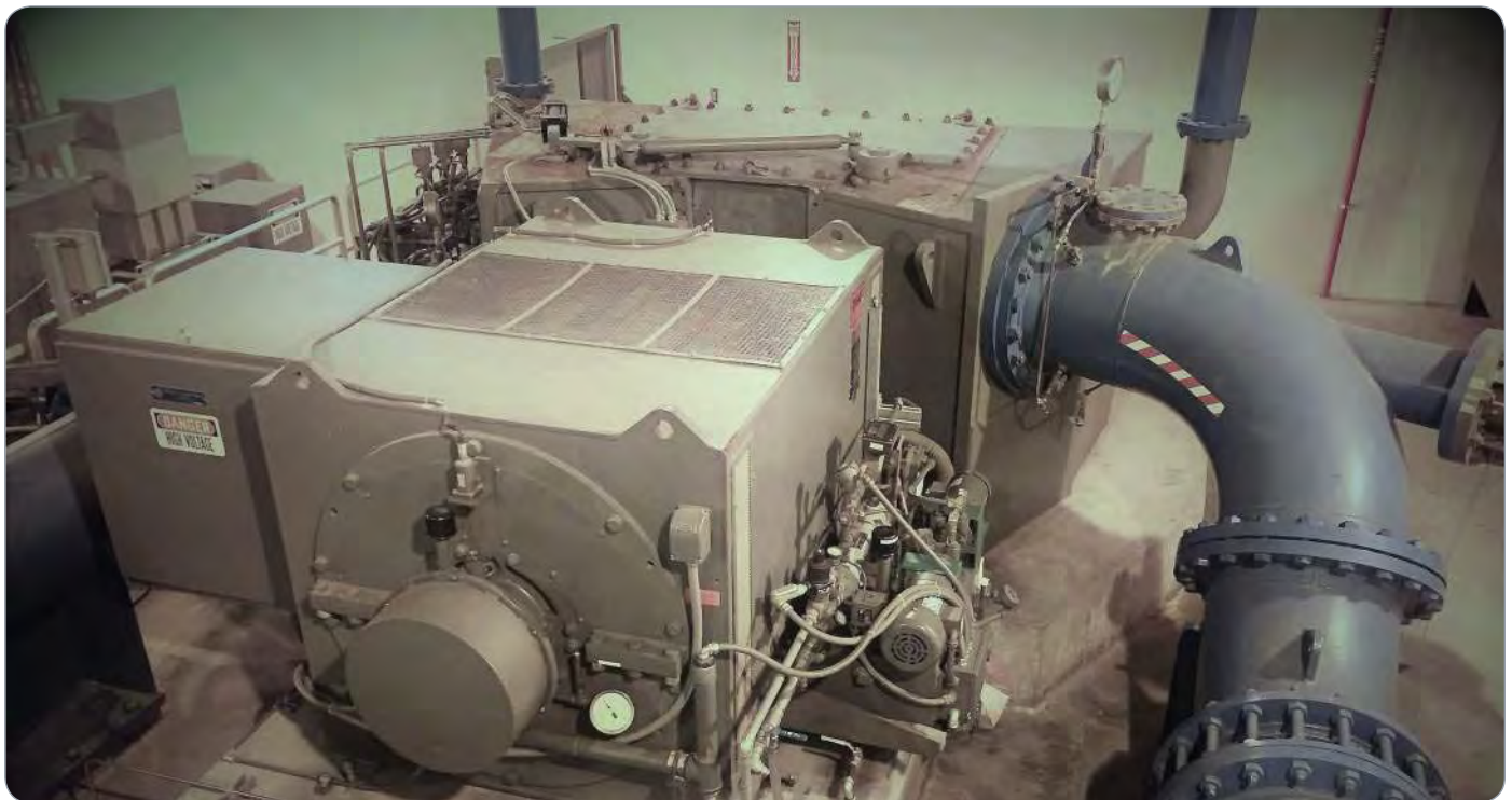
Eklutna Water Treatment Plant Turbine
