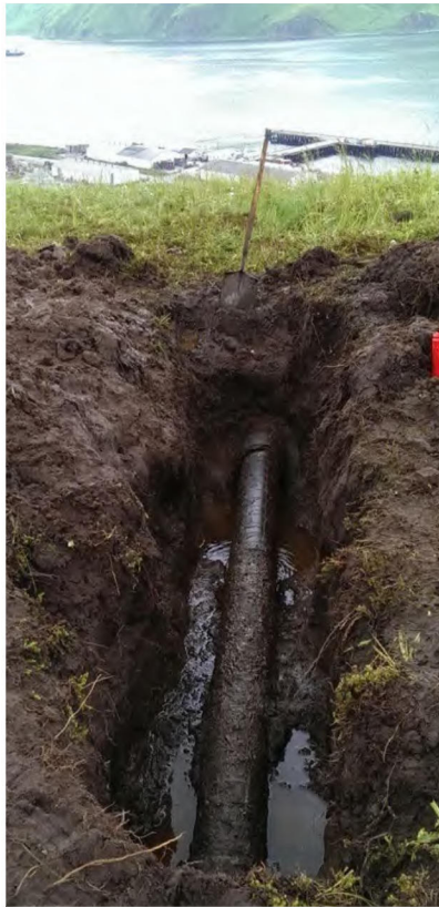
Figure 2: Leaking wood stave pipe connection to NPF (credit City of Unalaska)
