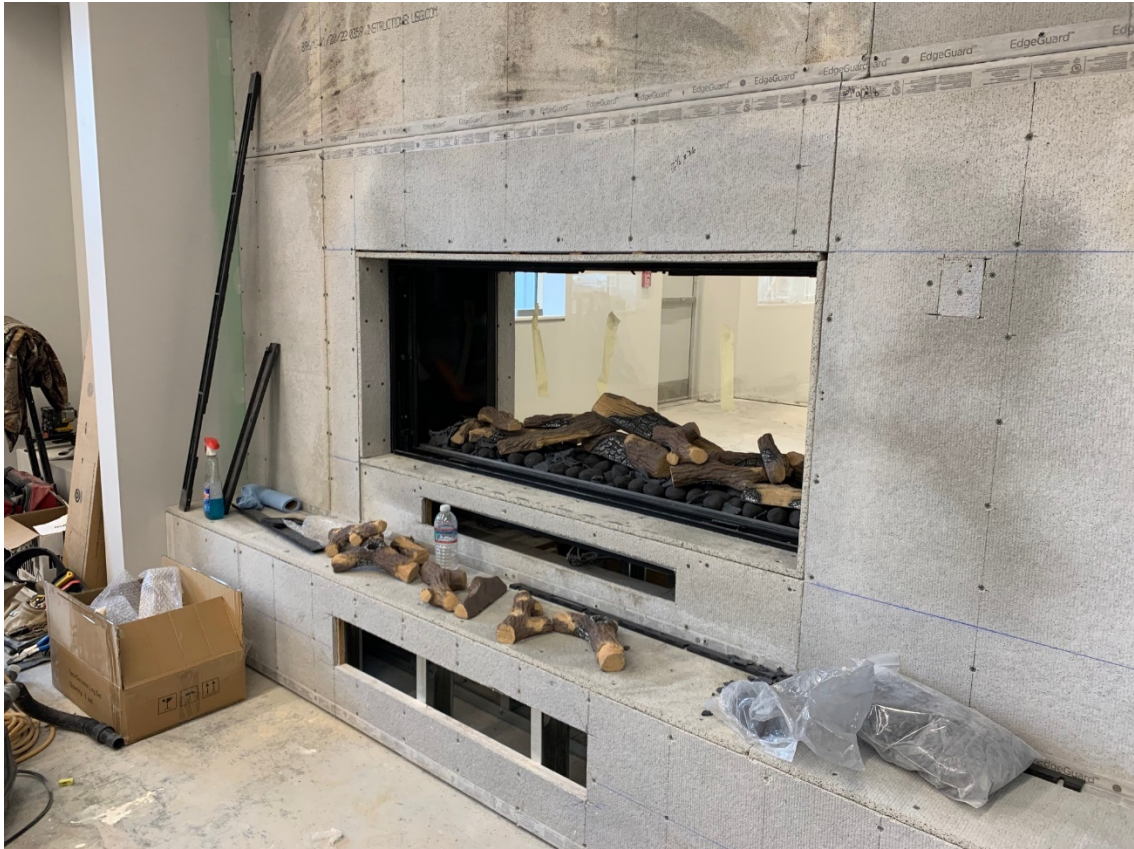
Fireplace Installation. When construction is complete, the fireplace will have a tile surround, with a woodblock collage by artist Ray Hudson. Photo by F&W Construction.
