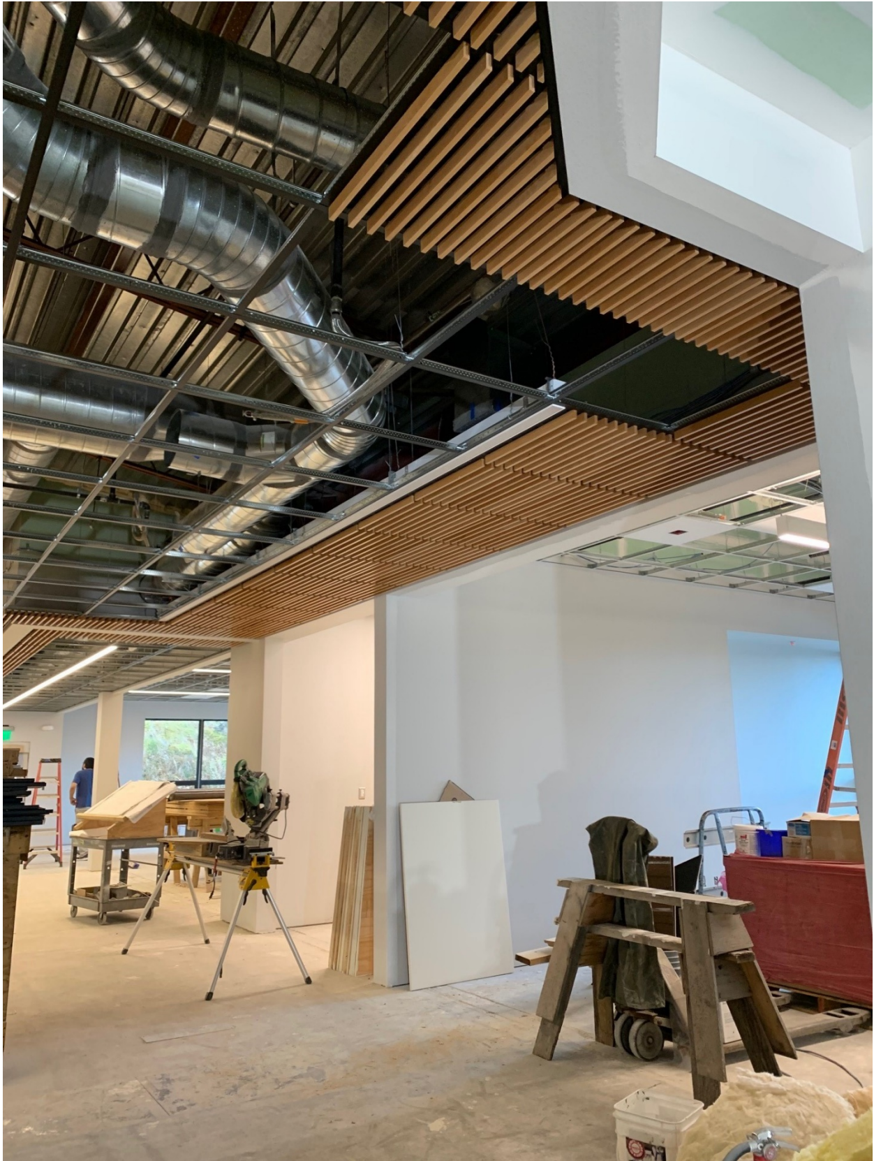
Interior view shows new paint, lighting, and ceiling panels. The children's room is partially visible on the left. A study room is in the center, and the teen room is on the right. These areas are largely inside the expanded square footage. Photo by Karen Kresh, City of Unalaska.
