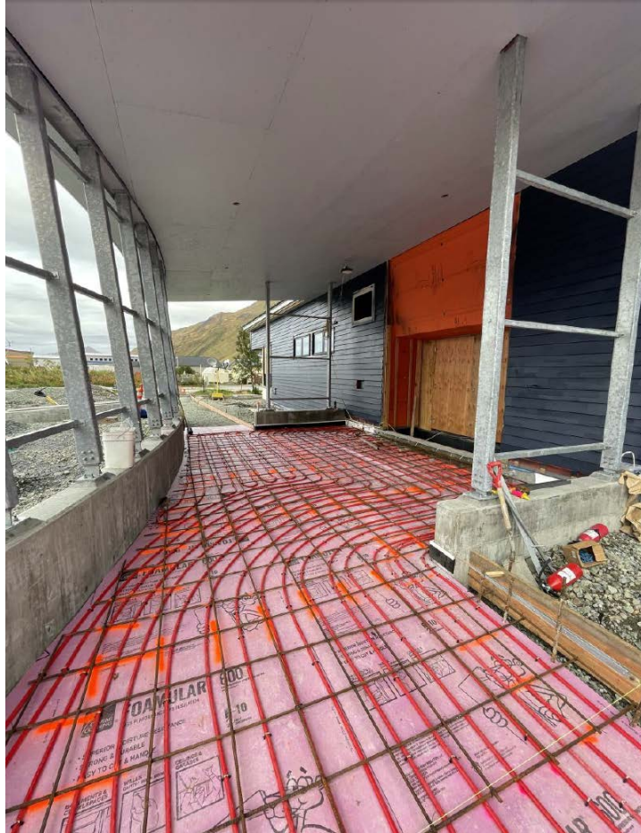
Entryway before final concrete pour, with visible rebar and icemelt system tubing. Photo by F&W Construction.
